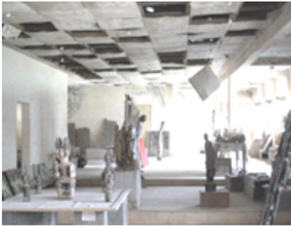
Fig. 5. The Ceiling of the Museum falling off
